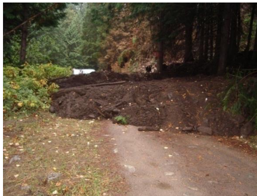
Photo 7 N Ent 2 part of debris flow deposit
