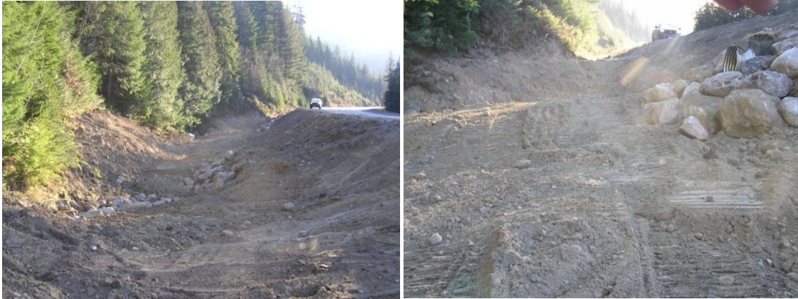
Photos 13 and 14 Additional debris flow storage volume and new overflow culvert installation above highway near middle Van Tuyl Creek
