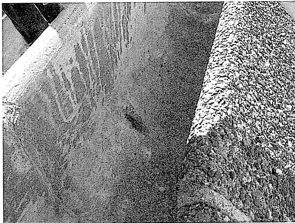
Photos 3 & 4: Swimming Pool pre-cast gutter deterioration
